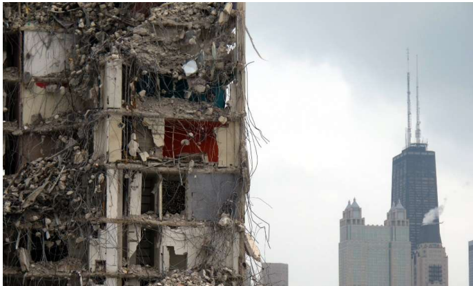
The demolition of Cabrini-Green, with Downtown Chicago in the background, image courtesy of Joe M500 via Wikimedia Commons
